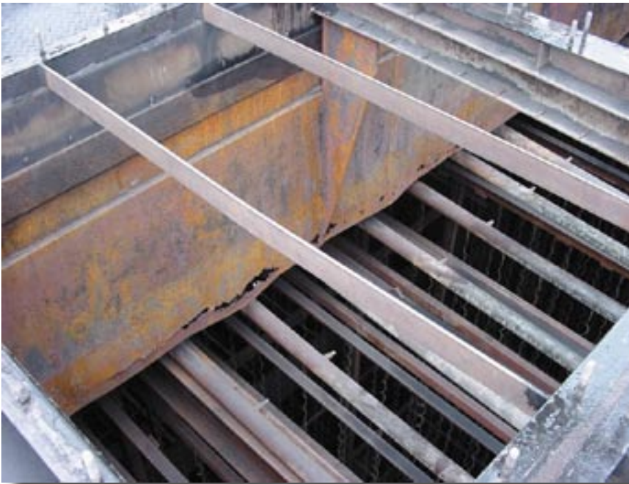
Figure 5. Severe corrosion in an electrostatic precipitator.
