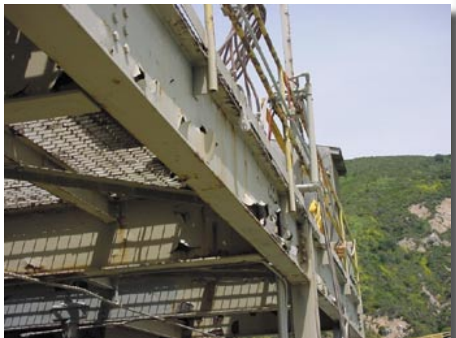
Figure 6: Severe corrosion of structural steel.
