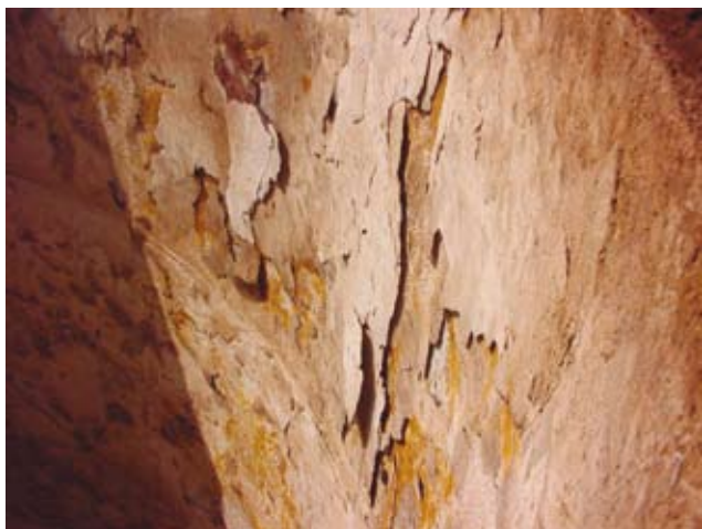
Figure 2. Rust scales inside a chimney.
