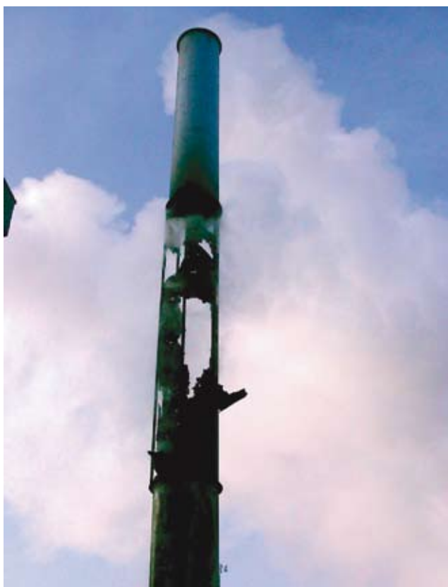
Figure 4. A severely damaged chimney.
