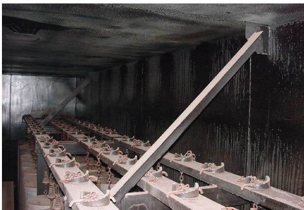
Figure 9. Inspection of FlueGard-225SQC after five years in a baghouse filter, showing no corrosion.
