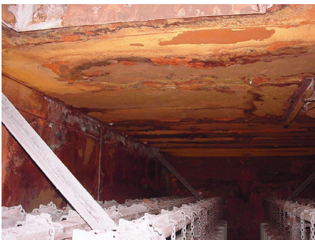
Figure 2. Severe corrosion damage in a reverse air baghouse filter.
