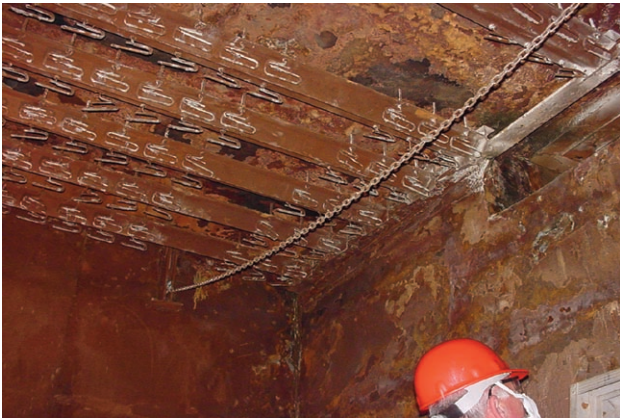
Figure 3. ESP walls made of SS304, corroding severely.
