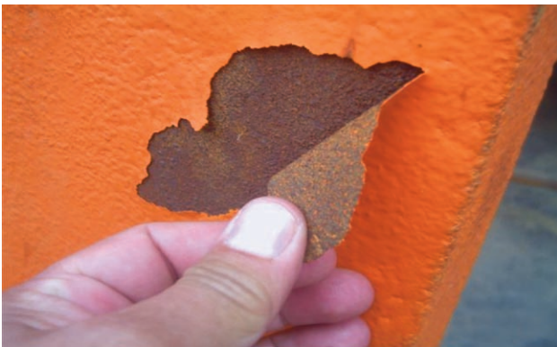
Figure 4. Blistering and delamination of an epoxy coating.
