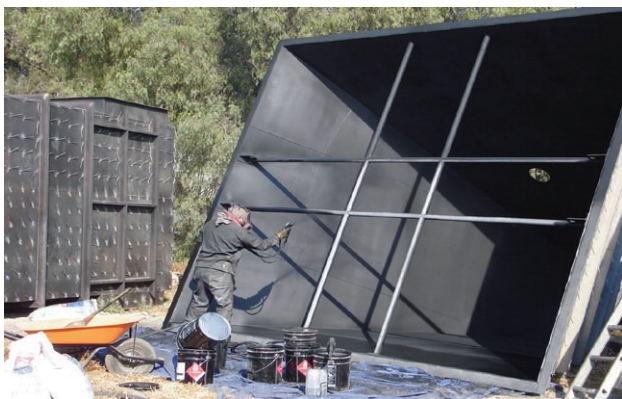
Figure 10. New baghouse filter coated with FlueGard-425S and cured at 200 °C.
