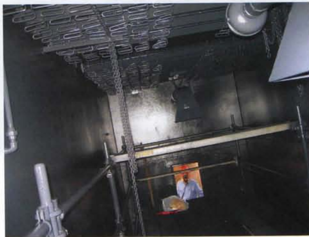
Figure 5. Coating of a baghouse in California.
