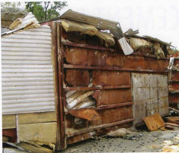
Figure 3. Severely corroded baghouse filter after three years.
