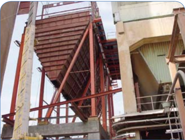
Figure 3. New ESP filter in Mérida, México, coated with FlueGard-225.
