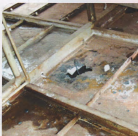
Figure 5. Roofing corroded due to refractory failure.
