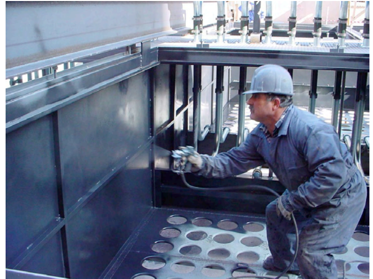
Baghouse Filter Protected with FlueGard ® -225SQC
