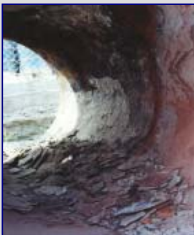
Corrosion in a duct
