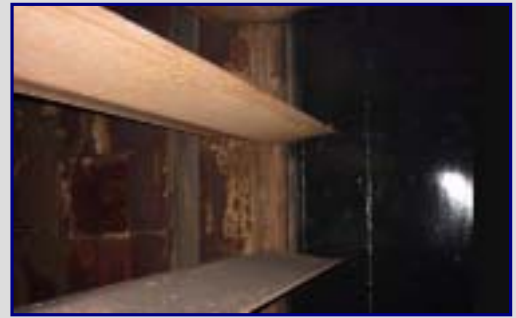
Left side corroded, right side coated
