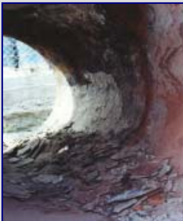
Corrosion in a duct
