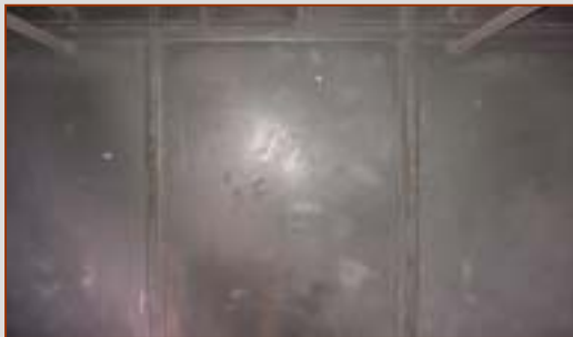
New baghouse coated, one year later
